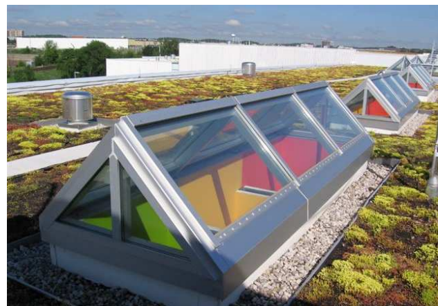
Figure 9-38: Green roofs are an effective stormwater best management practice and contribute to the reduction of the urban heat island effect.
