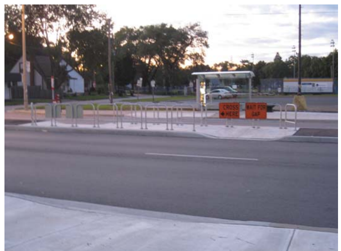
Figure 3-37 A centre median treatment intended to increase pedestrian safety, complete with curb ramps, signage and railings.
